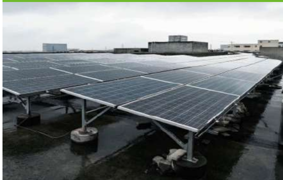
Solar Photovoltaic Power Generation System
